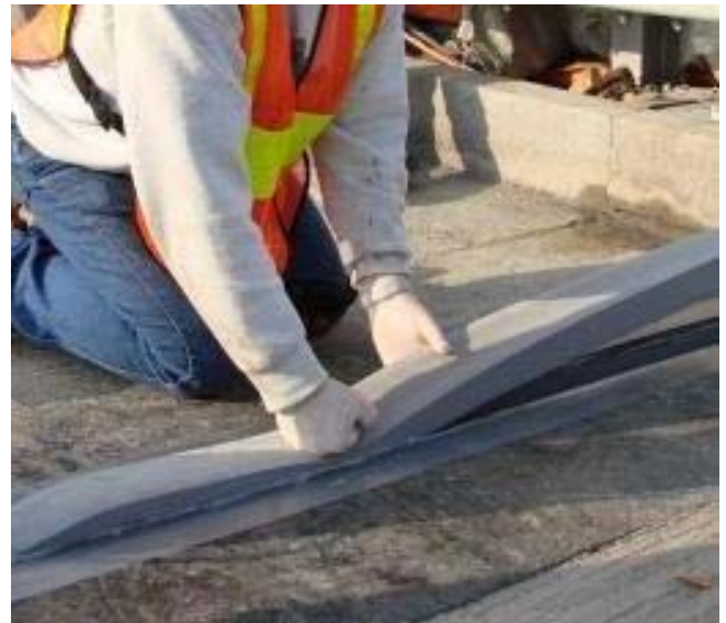
Starting the 'Tail' Dry. Tape down protection on the concrete surface prior to mixing Pro-Bonder to minimize cleanup.
